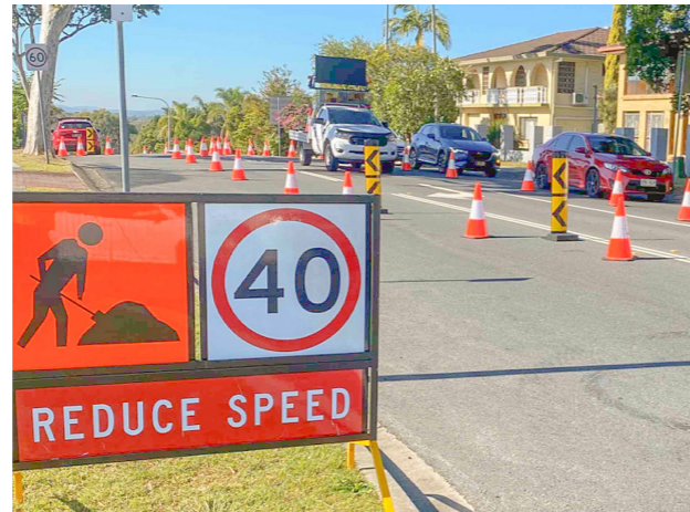
Long-term signage helps maintain safety and assist with the flow of traffic even when traffic controllers are not present on site, ie when works are expected to take over a day to complete.
