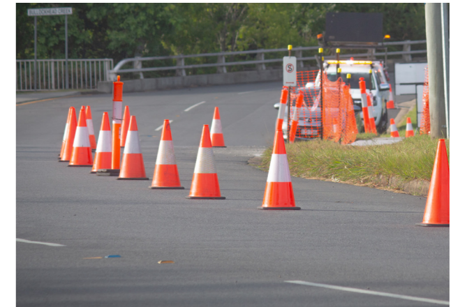
Traffic control trucks can help assist drivers by warning them well in advance that there are road works in progress ahead.
